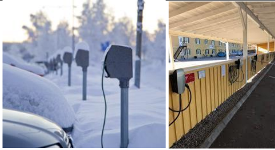
Electricity post for car engine heaters.
